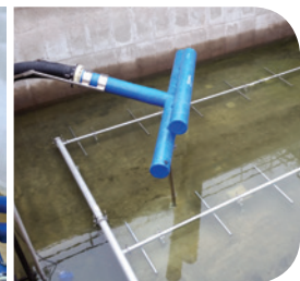
Fixed Diffused Aeration
